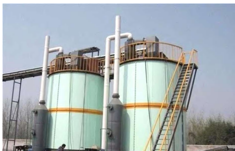
Figure 10. Tower composting equipment.
